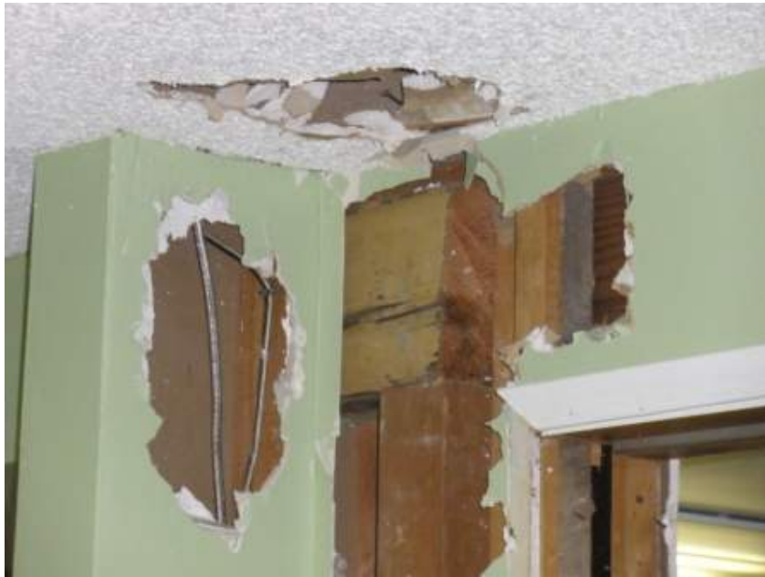
damaged ceiling material
