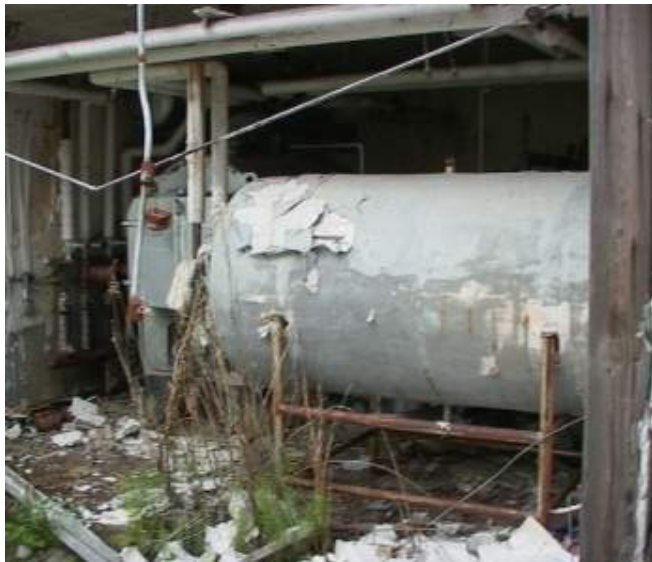
Asbestos insulated boiler
