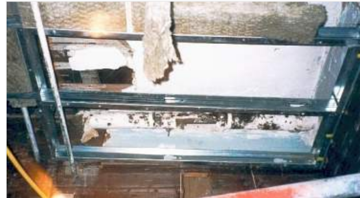
Damaged asbestos pipe insulation
