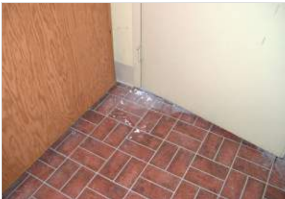
Asbestos debris on floor
