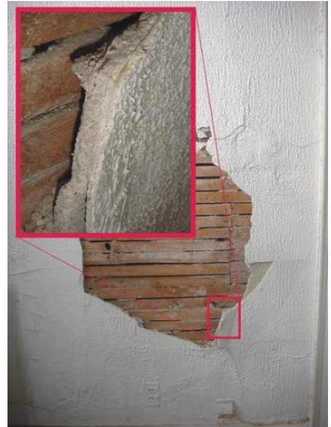
Plaster with asbestos
